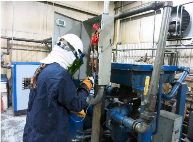
Tennessee Tech IAC student Melissa Moffet installs a data logger to measure and record electricity use of process equipment at a manufacturing facility in Tennessee.
