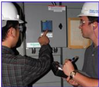
Fangxiao Dong and Jake Trimpe record voltage, amps, and current on an equipment display.
