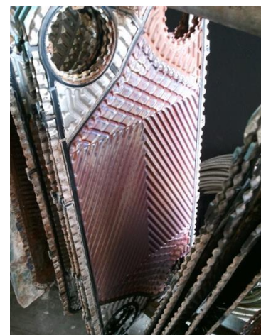
Inside of a plate and frame heat exchanger
