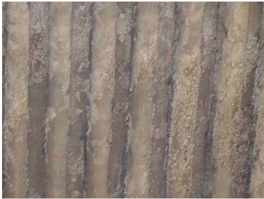
Results of poor water treatment.
