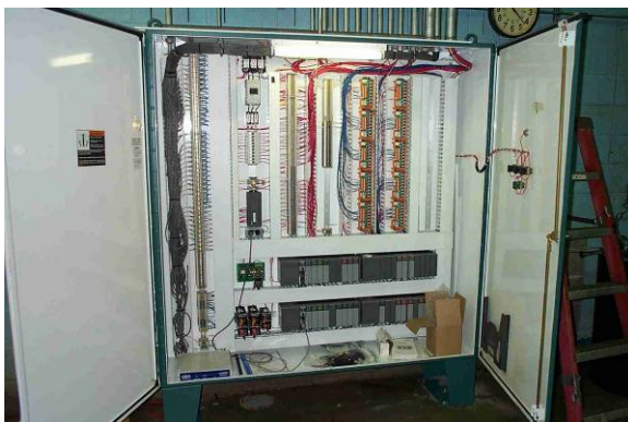
Sample control system I/O panel.
