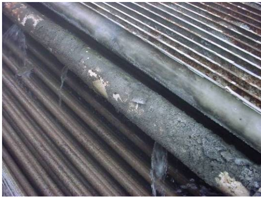
Plugged condenser nozzles.
