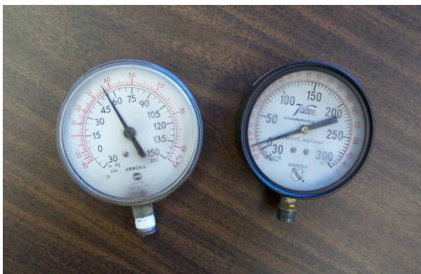
Faulty mechanical gauges.
