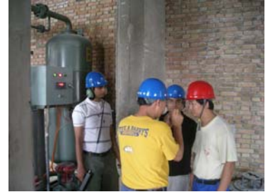
Dr. Gopala and Subodh working on a compressed air system in New Oriental Aluminum facility in China.
