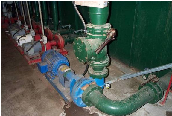
Sample remote condenser pump.
