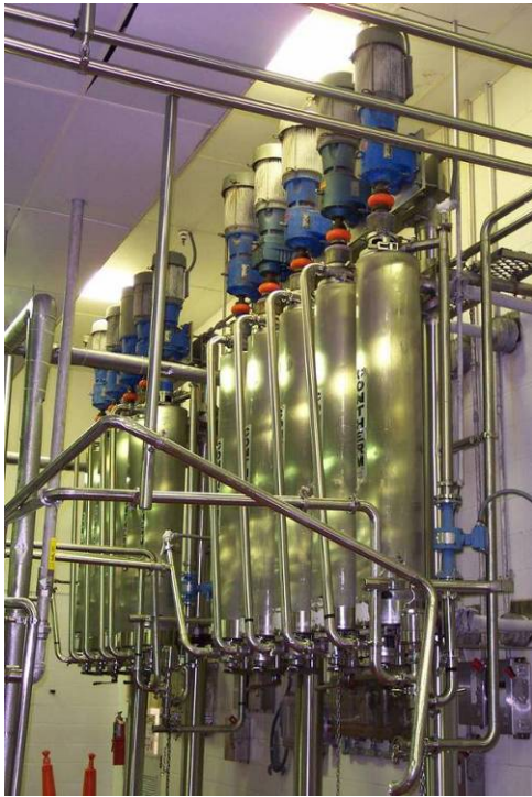
Multiple suctions on heat exchangers.
