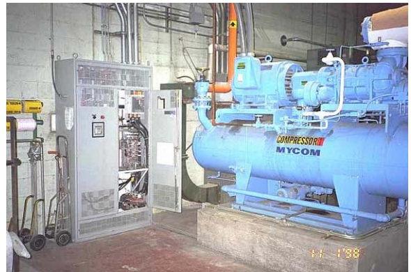
Sample compressor VFD application.
